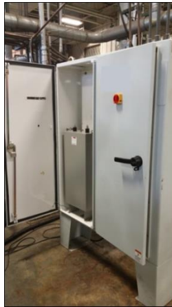
Figure 6. NEMA 12 Cabinet Housing the Components of the Power Supply (the main capacitor is shown)
